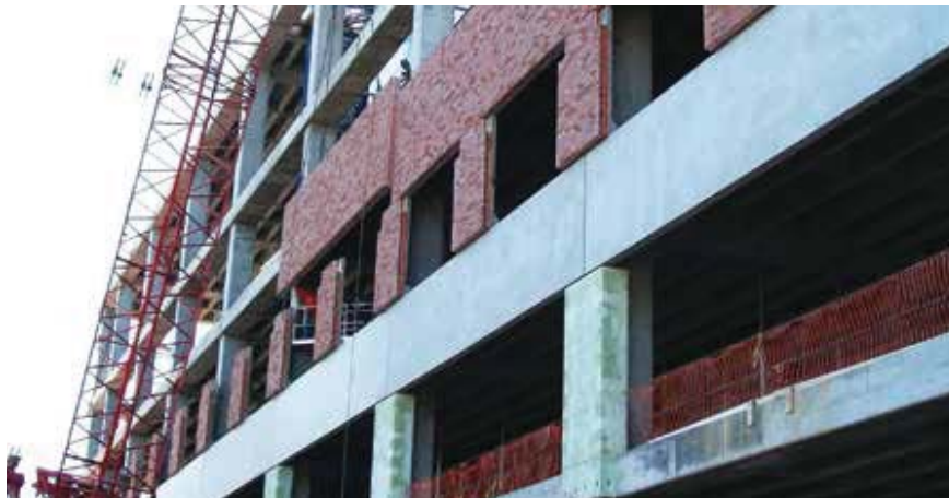
Only 24 weeks were required to erect the entire structure, including both the podium or base section and the towers. Photo: Gate Precast Co.
